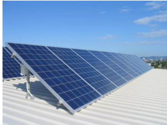
Figure 27: Example of Roof-Mounted Solar Array
